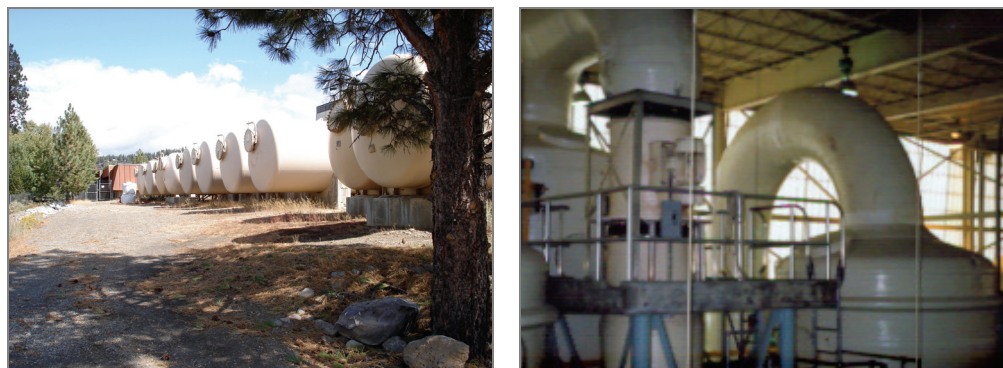
Fig. 3. Natural clinoptilolite columns for ammonium removal and the inside of the regeneration hall at Tahoe Truckee Sanitation Agency in California
